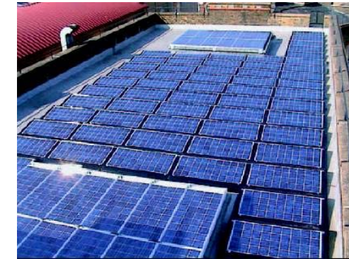
Figure C3 Solar PV panels. PV panels angled at 10° on flat roofs
