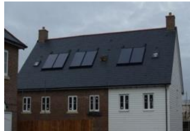
Figure C2 Solar hot water installation. Schuco flat plate system providing domestic hot water ( photo courtesy of Ecolution Renewables)
