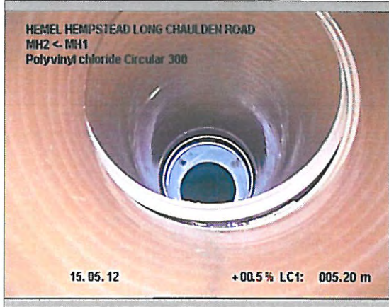
Photo: 3_3A, 00:00:55 5.2m, Joint displaced, large
