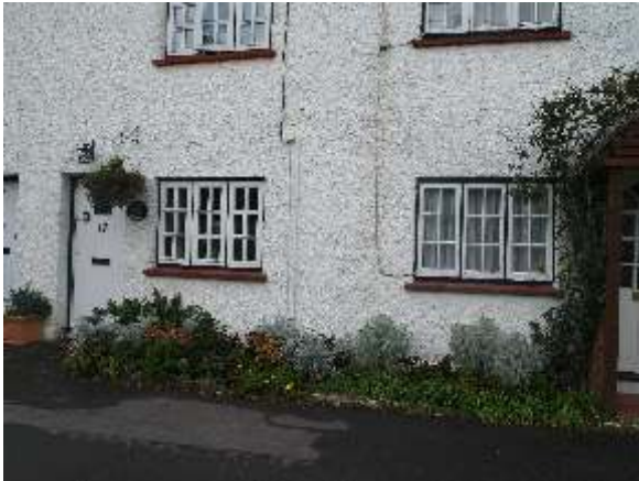
Inappropriate replacement windows here upset the rhythm of traditional cottage fenestration
